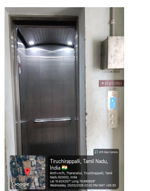
Lift in Controller of Examination
