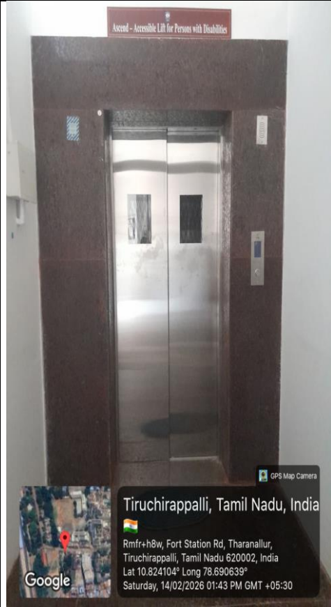
ASCEND Lift in Rehab Block
